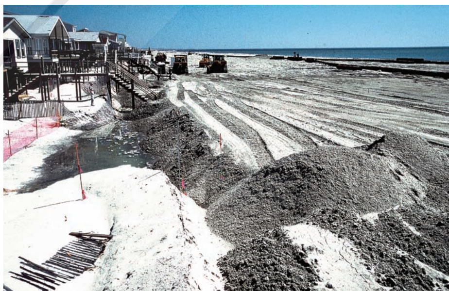
▶ FIGURE 13-29. To replenish a beach, the U.S. Army Corps of Engineers pumped a high volume sand-and-water slurry from up the coast in 30-inch pipes. Heavy earthmoving equipment spread more than a meter of sand across the new beach at Ocean Isle Beach, North Carolina, in March 2001.
