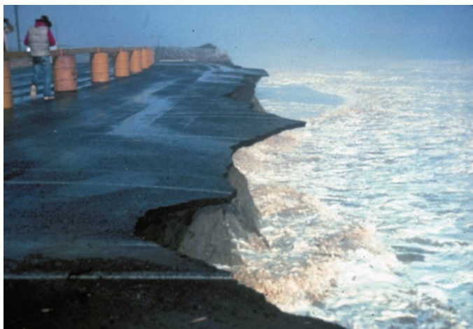
► FIGURE 13-26. Storm waves undercut this East Coast parking lot, causing it to collapse into the ocean.
