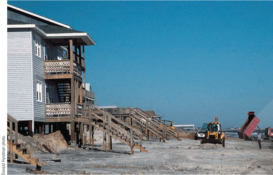
► FIGURE 13-28. A truck dumps rusty, fine-grained sand excavated from the lagoon side of a barrier bar at Holden Beach, North Carolina, following a small storm in March 2001. Such sand is more easily eroded by smaller waves than the natural sand on the beach.
